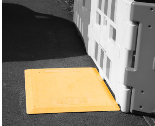
TRENCH COVER INSITU
